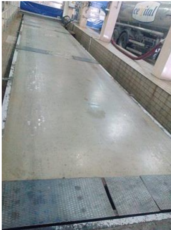
Figure I.6.2 Pont bascule ROC
