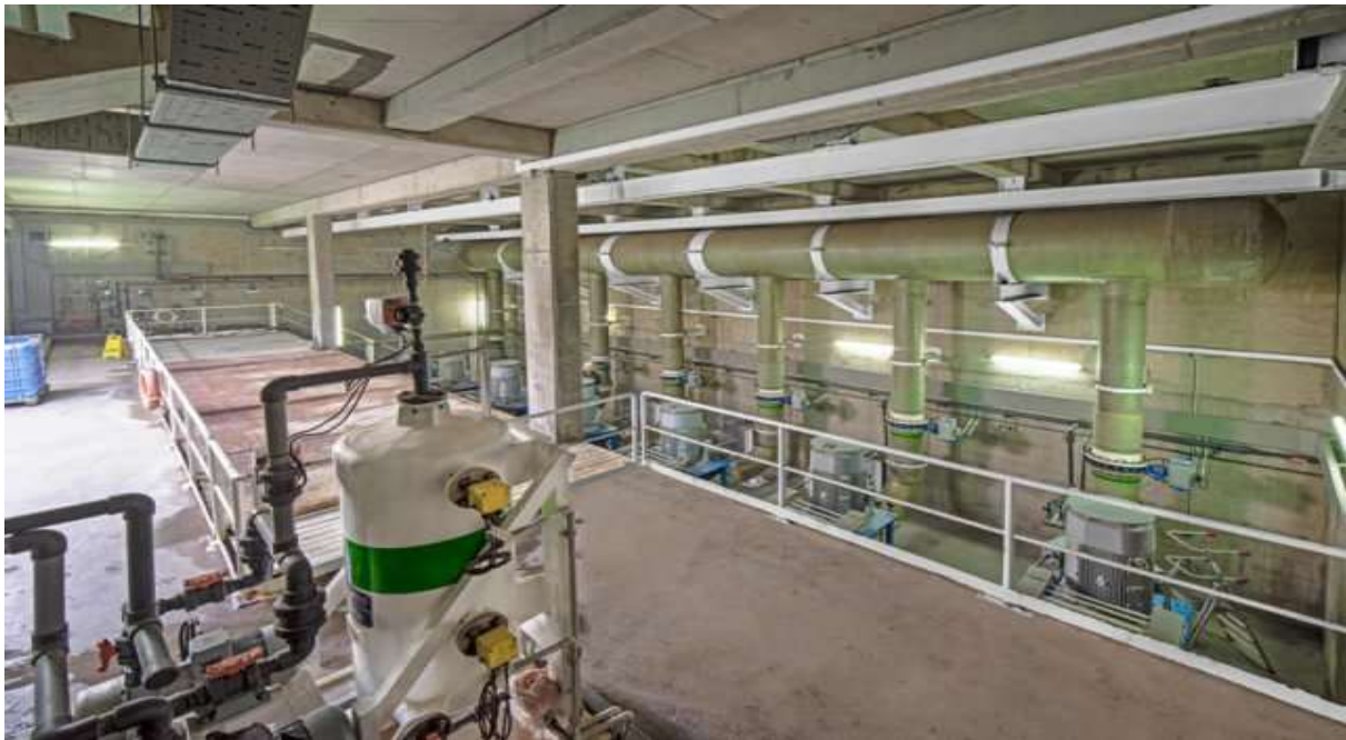
Figure II.3 : Station de pompage eau de mer
