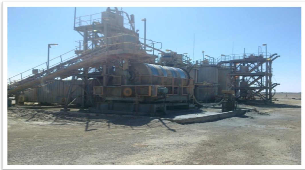
FigureII.8: Station de broyage. [Source : Photos prise]
