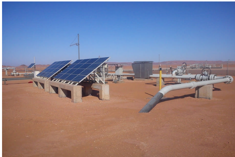
Figure (III.1). L'installation photovoltaïque TG:04 .
