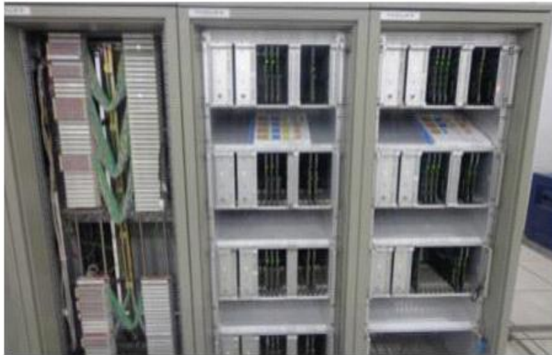
Figure (III.12): Armoire du VCC.
