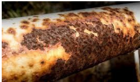
Figure I.10: Corrosion uniforme (What Is Corrosion & the 10 Most Common Types, 2025).
