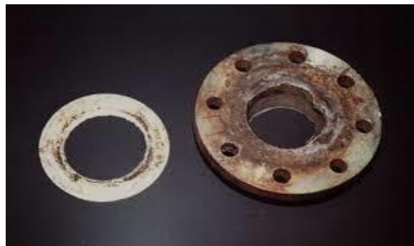
Figure I.12: Corrosion caverneuse (what does Erosion-Corrosion mean - AONG website, 2025).
