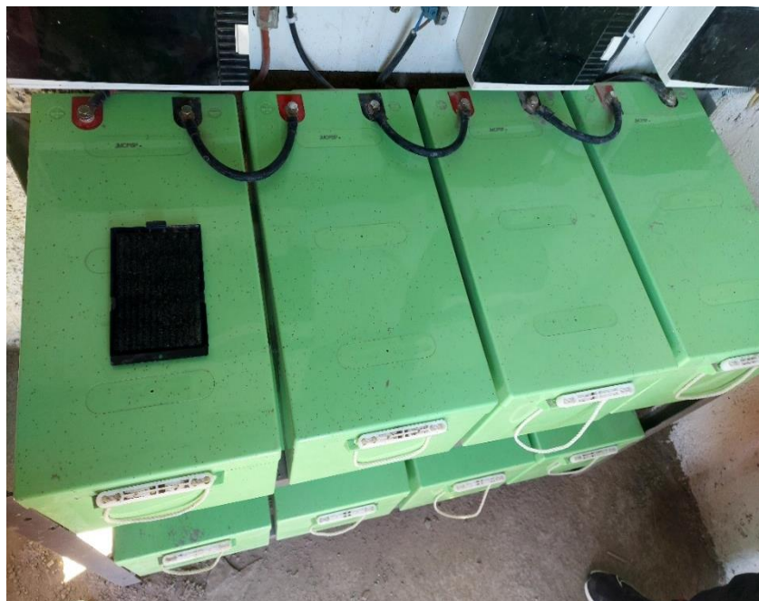
Figure III.12 : Raccordements des batteries
