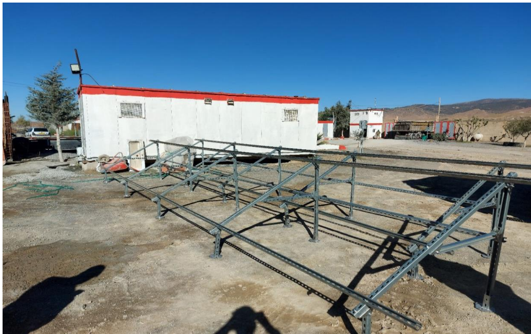
Figure III.5 : Structures porteuses des modules photovoltaïques
