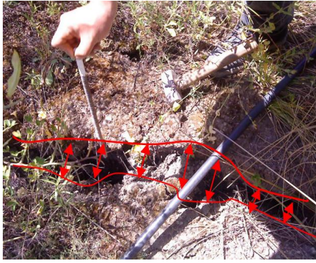
Figure 1.39 : Fissuration notable du sol
